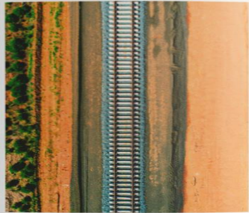
MAIN IMAGE An aerial view of the Inland Rail construction site showing the long, straight path of earth and gravel.
